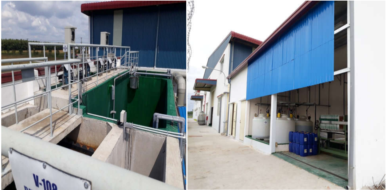
Wastewater treatment system at Yu Wei VN Co., Ltd - 150m 3 /day
