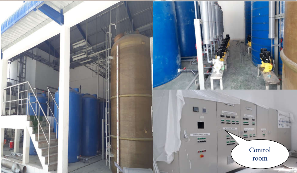
Wastewater treatment plant at Yue Chang VN Co., Ltd - 2000 m3/day
