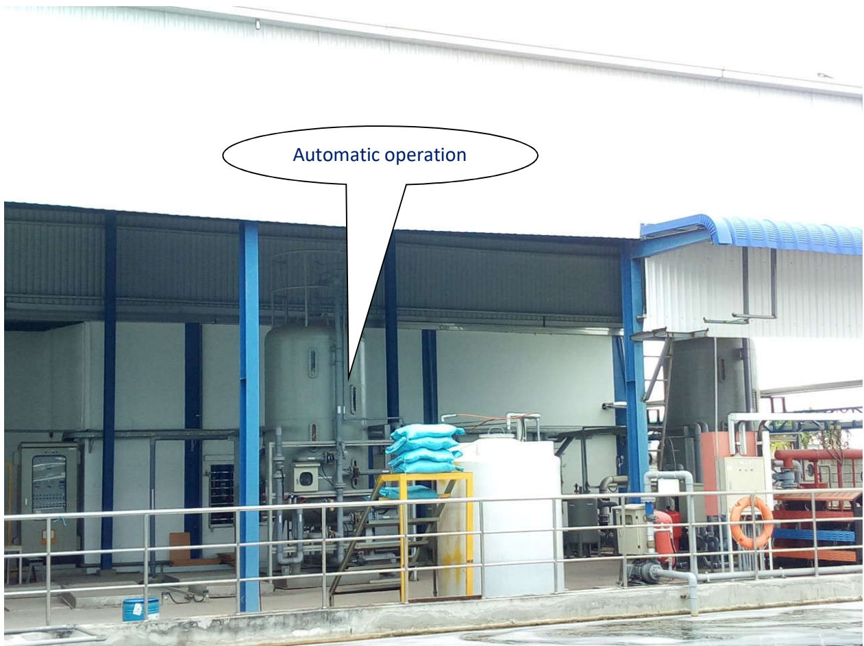
Softening water treatment system at Yue Chang VN Co., Ltd - 1000m 3 /day
